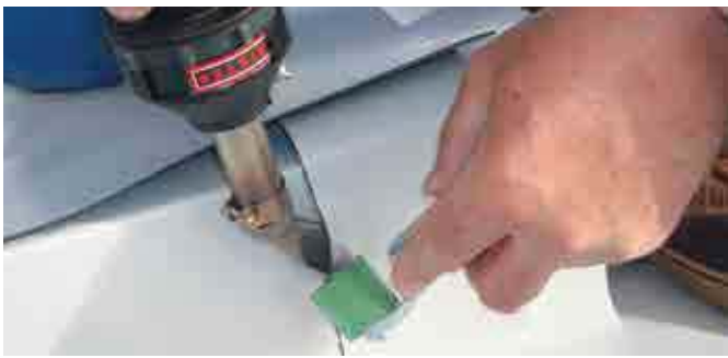
HOT JET S with angled nozzle welding a T-joint on the roof.
